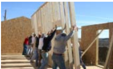
This could be you building a home on the Lakota Sioux Reservation in Eagle Butte, SD.
